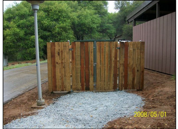
Enclosed Transformer at Madrone
