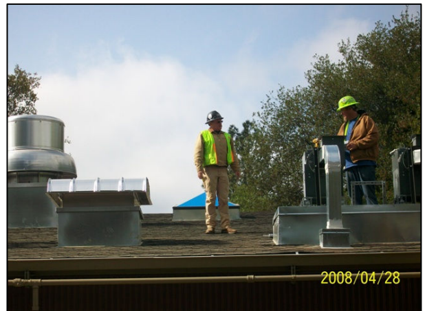
Connecting Roof Fans
