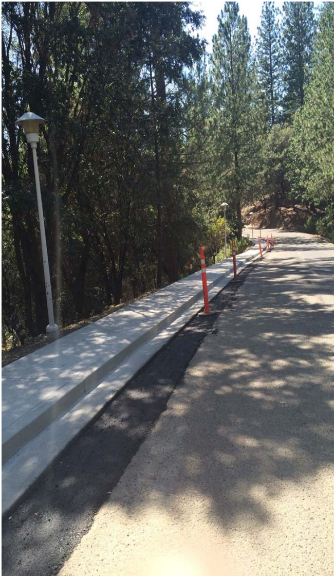
Asphalt fill at Columbia College Drive
