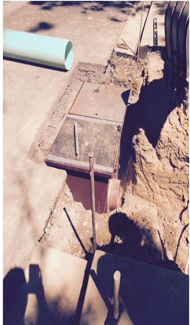
Storm water vault @ Willow
